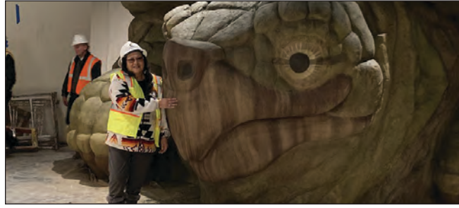
Photos Courtesy of Michael Hanke Sue Folsom during construction of the Children's Activity Room at the Choctaw Cultural Center.
