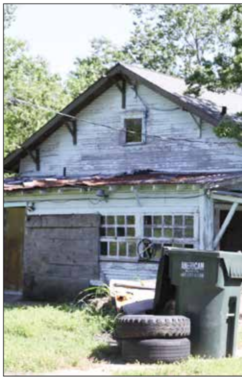
The Wilson's old home was in serious need of repair.
