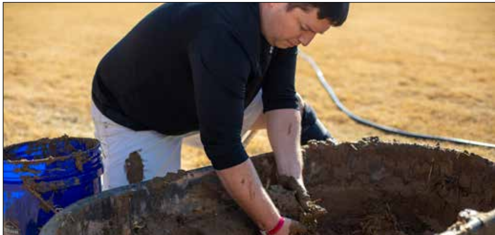
Stacey Fincher loads a bucket with the pre-mixed mud to place on the walls of the chukka.
